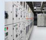
Low Voltage Switchgears
