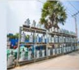
Single Phase Transformers
