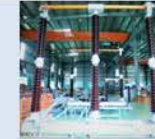
Disconnectors & by-pass switches
